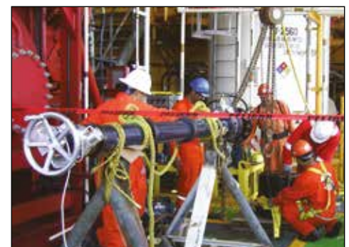
▼ CHT2000 hot tapping offshore application.
